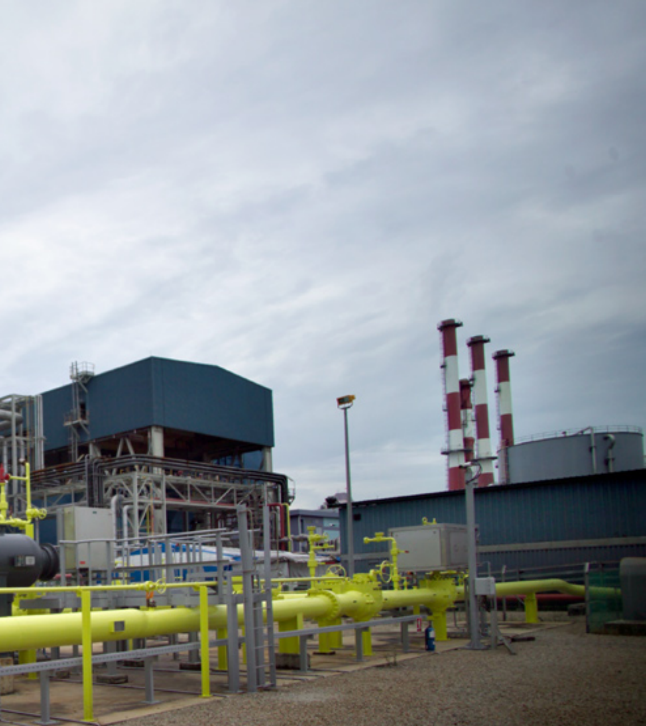
(Pictured) SembCorp Cogen, our gas-fired cogeneration plant in Singapore, receives piped natural gas from West Natuna, Indonesia.
