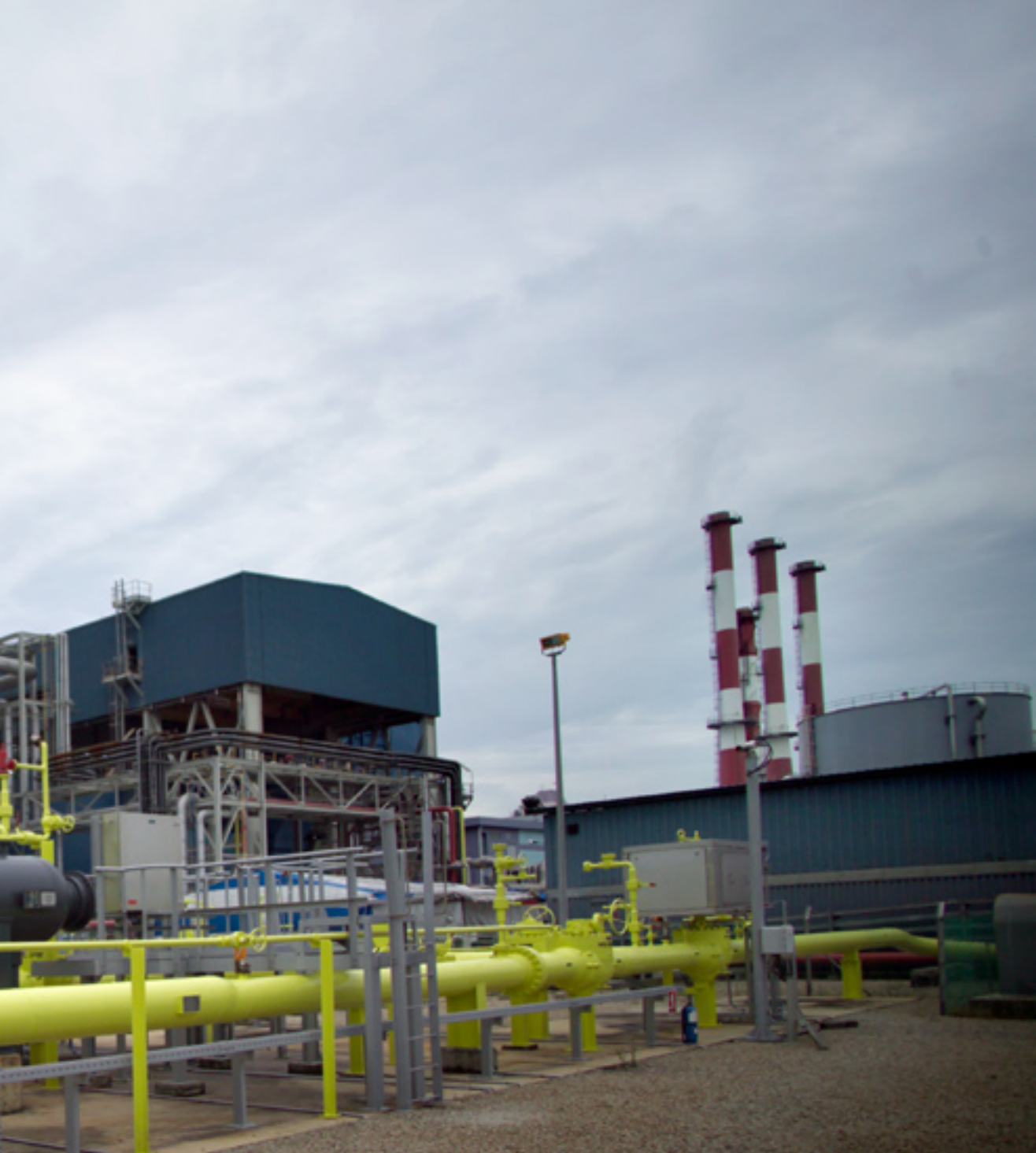
(Pictured) SembCorp Cogen, our gas-fired cogeneration plant in Singapore, receives piped natural gas from West Natuna, Indonesia.
