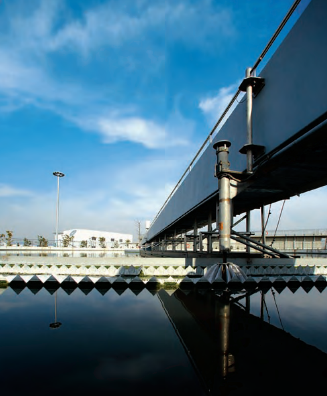
Semcorp's wastewater treatment plant in Nanjing Chemical Industrial Park in China.
