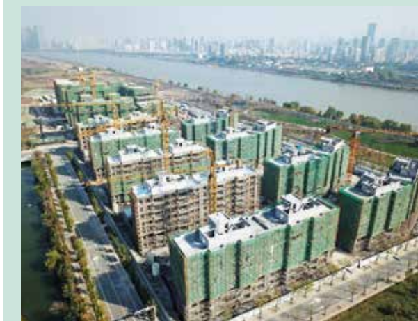
International Water Hub in China, a technology and business centre, as well as Riverside Grandeur, a residential development next door, celebrated their topping out in 2017. Both projects are on track to be completed in 2018
