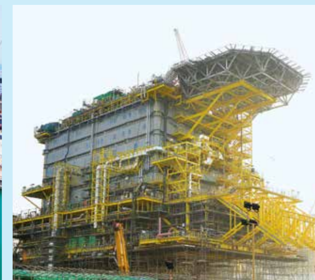
One of three topsides under construction for Maersk Oil. On completion, the topsides, comprising a central processing facility plus two connecting bridges, a wellhead platform and utilities and living quarters platform, will be installed in the Culzean field in the UK North Sea
