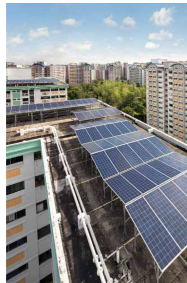
Sembcorp will build, own, operate and maintain grid-tied rooftop solar systems with a total capacity of 90 megawatt peak under the SolarNova programme
