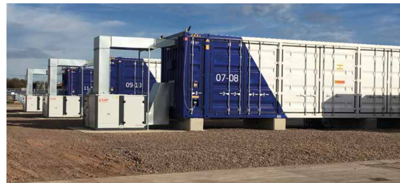
UKPR's 120-megawatt battery portfolio represents one of Europe's largest battery-based energy storage projects
