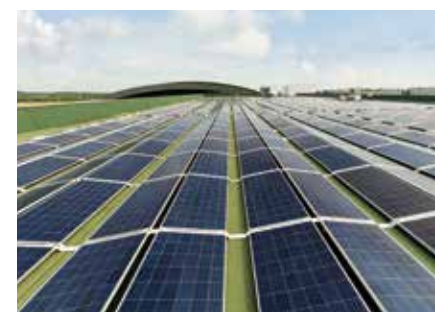
Secured additional 115 megawatt peak of solar power capacity since the end of 2017, becoming one of the leading solar energy players in Singapore
