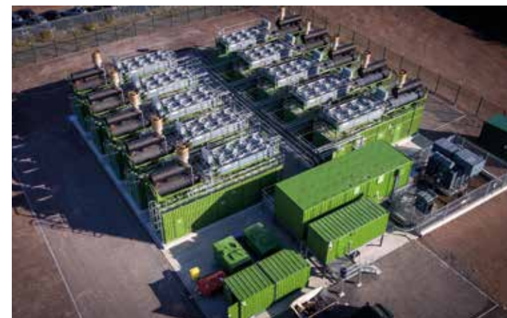
Deepened presence in the UK with the acquisition of UK Power Reserve (UKPR), the country's largest flexible distributed energy generator
