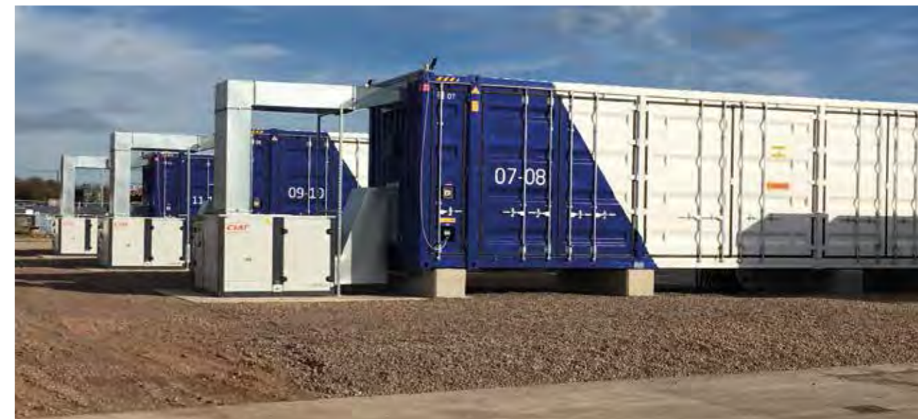
UKPR’s 120-megawatt battery portfolio represents one of Europe’s largest battery-based energy storage projects
