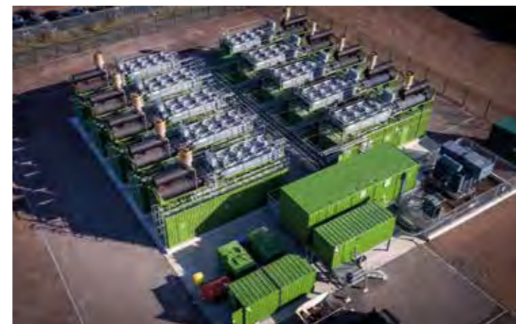
Deepened presence in the UK with the acquisition of UK Power Reserve (UKPR), the country's largest flexible distributed energy generator
