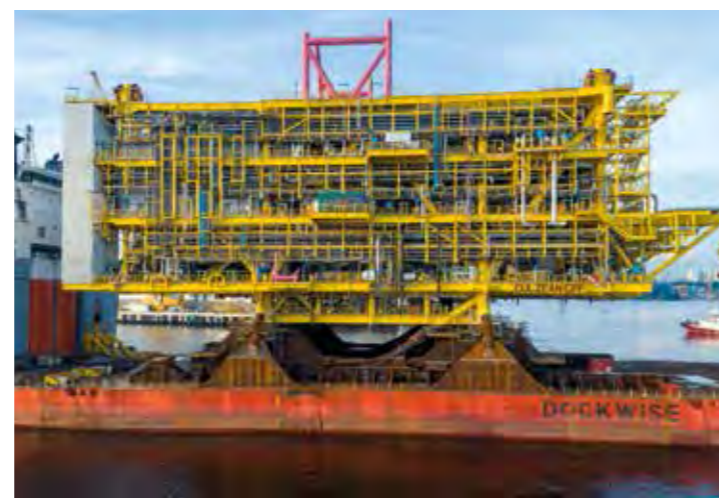
Delivered to TOTAL, this project involved the construction of wellhead, utilities and living quarters as well as central processing facility (pictured), for deployment in the Culzean field in the UK North Sea
