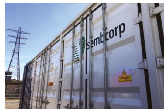
Sembcorp Energy UK's flexible gas-fired generation plants (top) and battery energy storage system (above)
