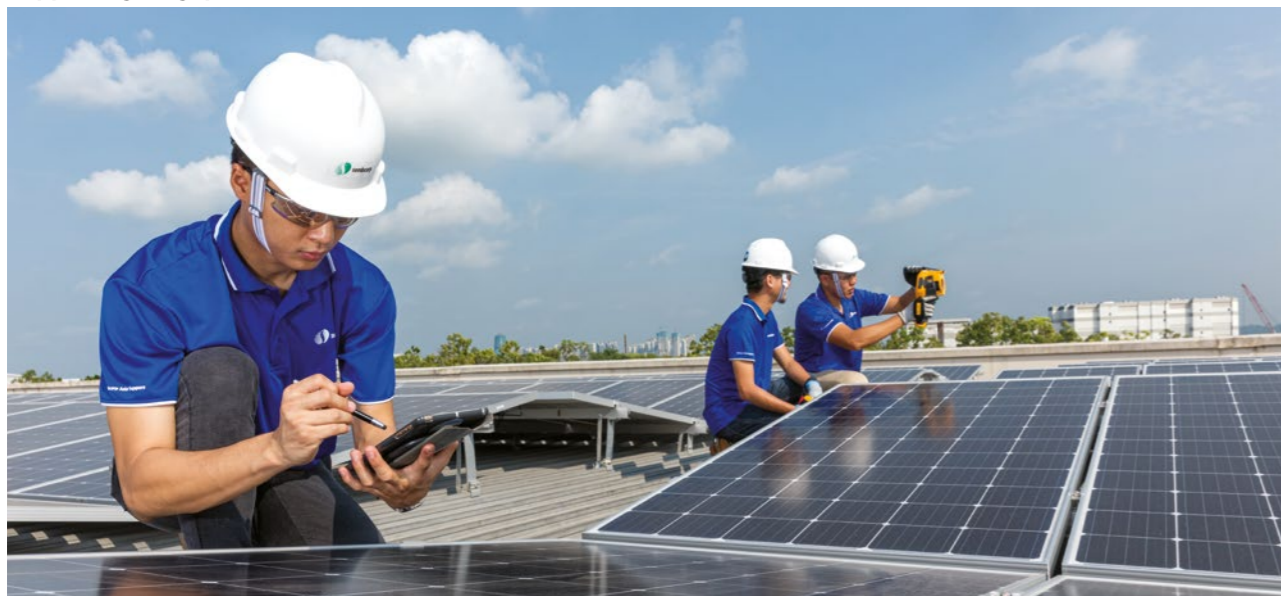
Sembcorp Solar staff inspecting our rooftop solar panels
