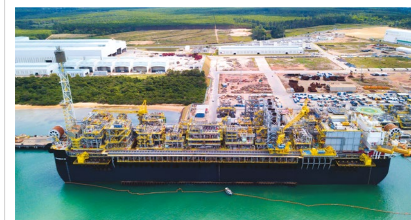
Topside modules construction and integration for the FPSO P-68 delivered to Petrobras, a testament to Estaleiro Jurong Aracruz's engineering, procurement, construction and commissioning capabilities
