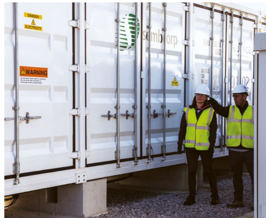
In 2019, we commissioned the first 60MW of our 120MW battery storage system in the UK, one of the largest fleets of its kind in Europe
