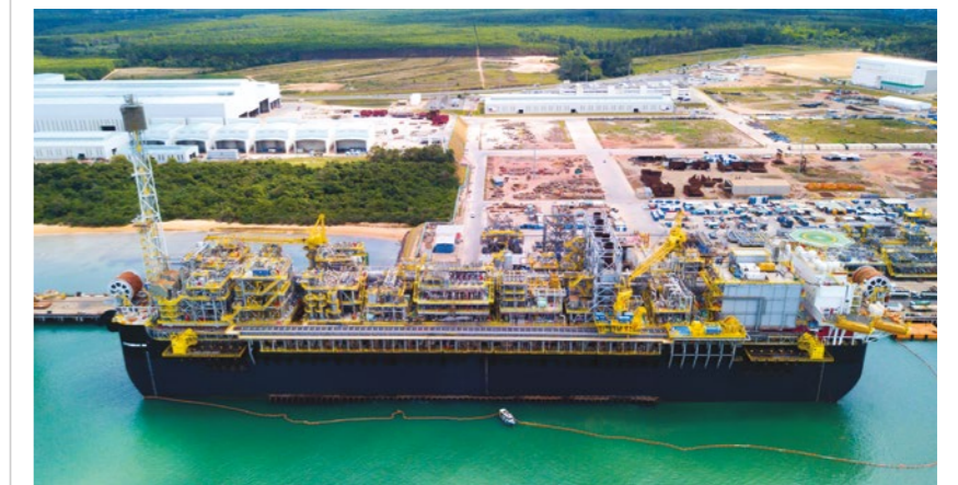
Topside modules construction and integration for the FPSO P-68 delivered to Petrobras, a testament to Estaleiro Jurong Aracruz's engineering, procurement, construction and commissioning capabilities
