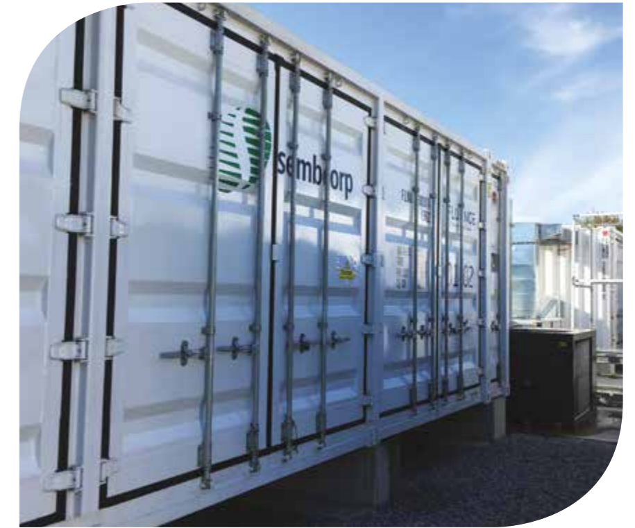
A further 60MW of our 120MW battery storage system in the UK will commence operations in 2021
