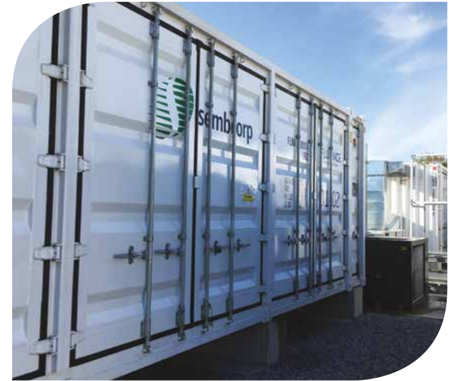
A further 60MW of our 120MW battery storage system in the UK will commence operations in 2021
