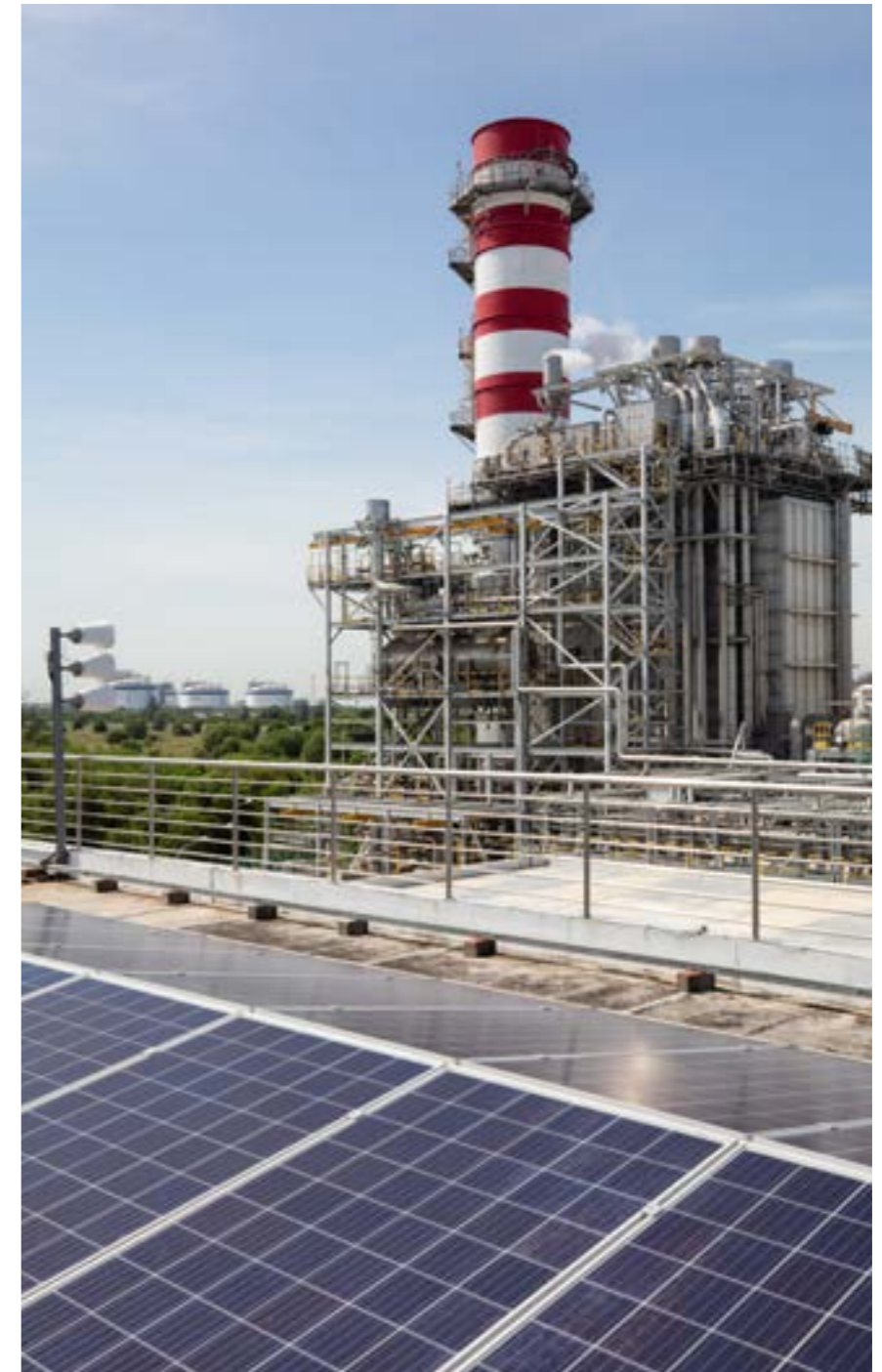
>> Sembcorp Cogen @ Banyan and solar panels installed on the rooftop of one of Sembcorp's facilities on Jurong Island, Singapore
