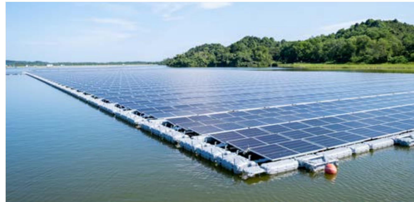
>> The Sembcorp Tengoh Floating Solar Farm, one of the world's largest inland floating solar photovoltaic systems
