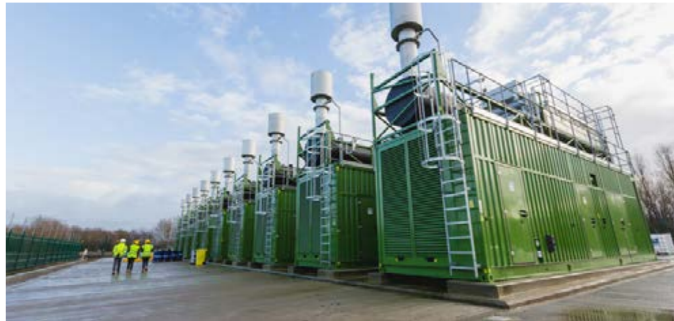
>> Sembcorp's flexible generation assets in the UK
