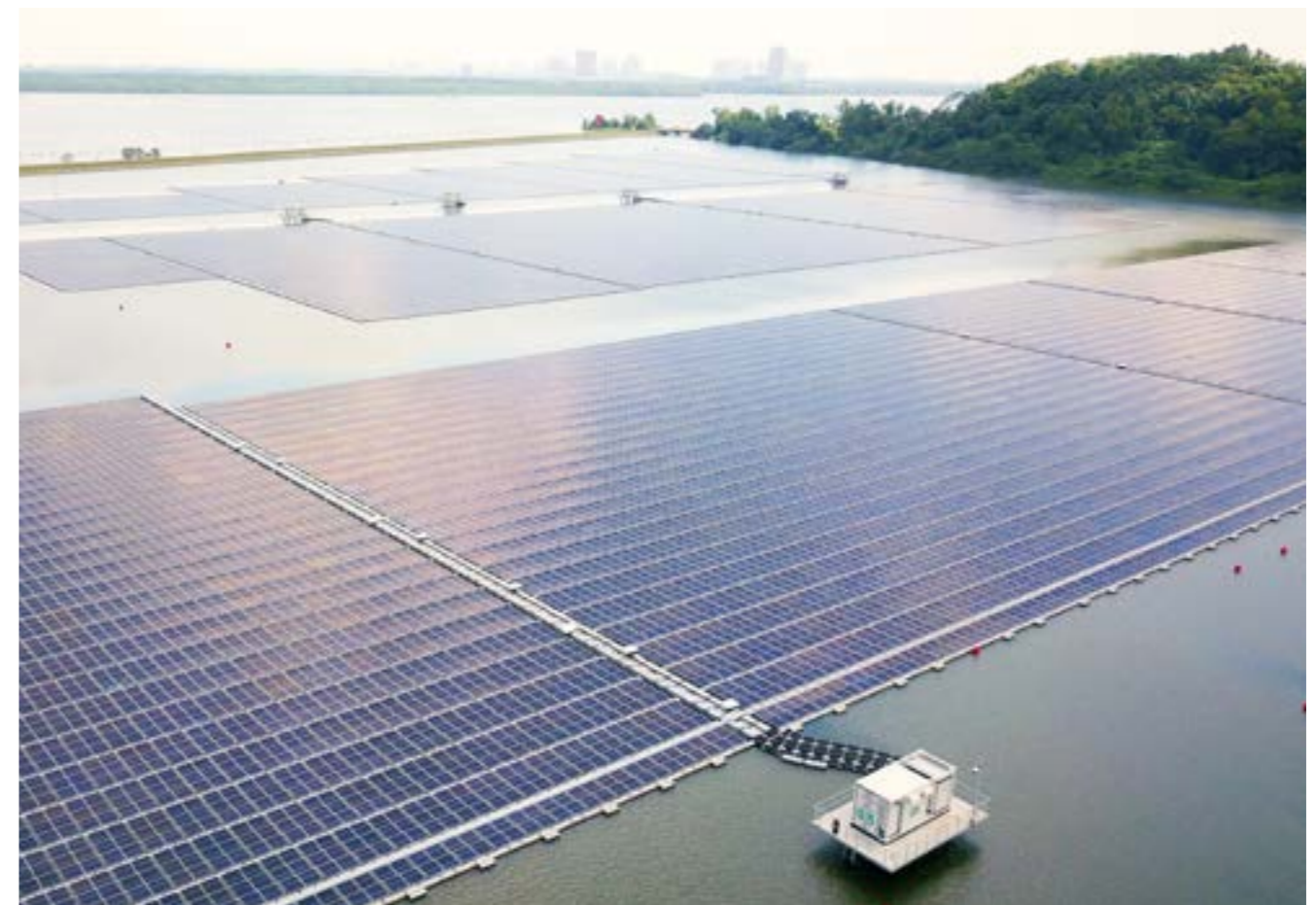
>> The 60MWp Sembcorp Tengeh Floating Solar Farm in Singapore, one of the largest inland floating solar farms in the world
