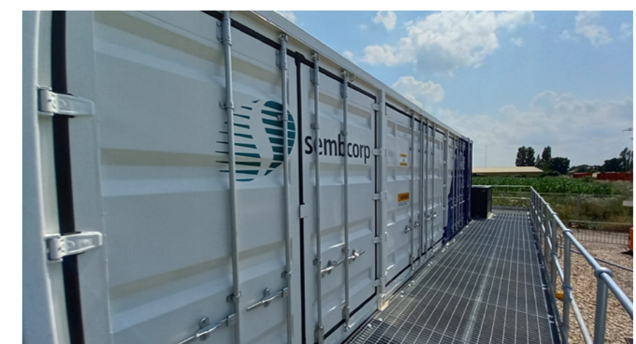
>> The remaining 50MWh of our 120Wh battery storage system in the UK will commence operations in 2022
