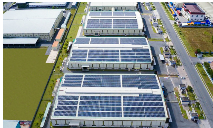
>> Sembcorp's Vietnam-Singapore Smart Energy Solutions installed rooftop solar systems at H.B Fuller in VSIP Binh Duong
