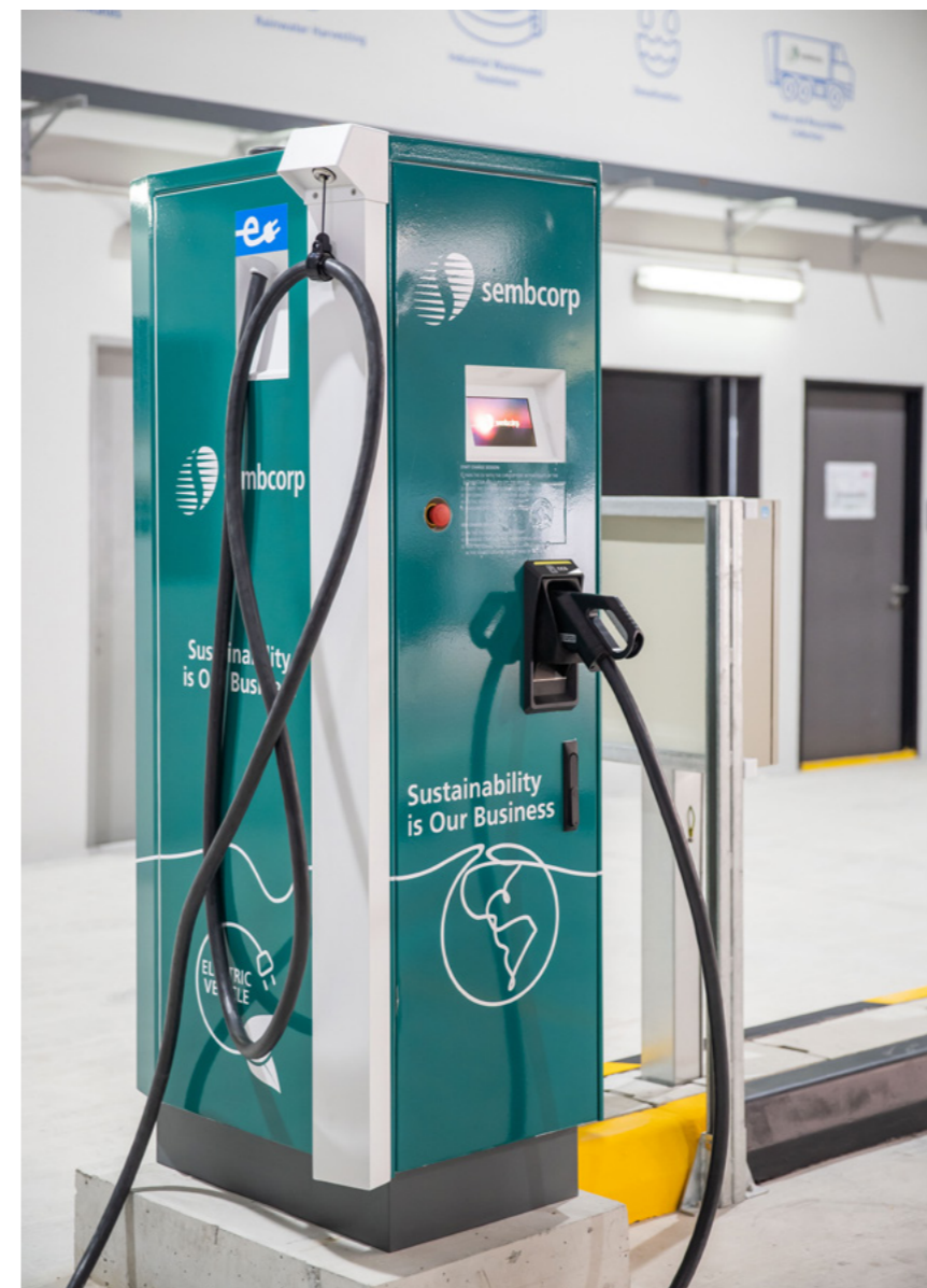
>> Sembcorp opened Singapore's first solar-powered electric vehicle charging hub at its Tuas depot in July 2021
