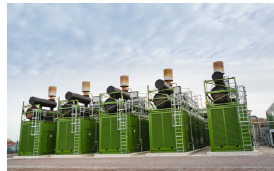
Sembcorp's flexible generation assets in the UK
