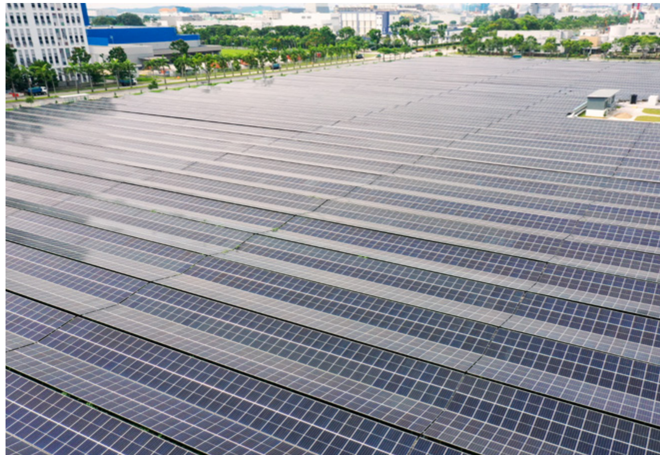
Sembcorp's solar farm in Tuas, Singapore's first solar farm with an integrated rainwater harvesting system
