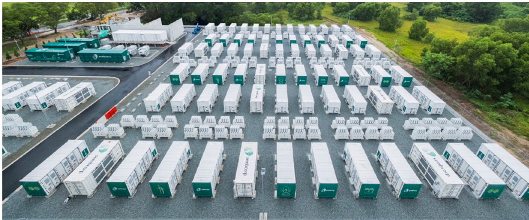
Sembcorp is one of Asia's largest ESS operators with a battery storage portfolio of 501MW / 709MWh in Singapore and the UK
