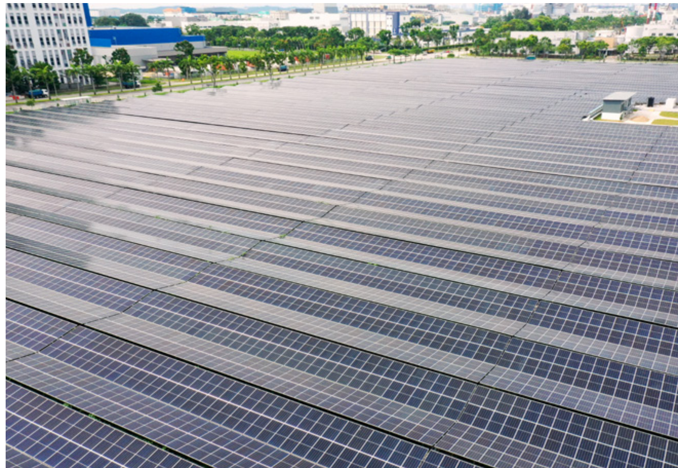
Sembcorp's solar farm in Tuas, Singapore's first solar farm with an integrated rainwater harvesting system
