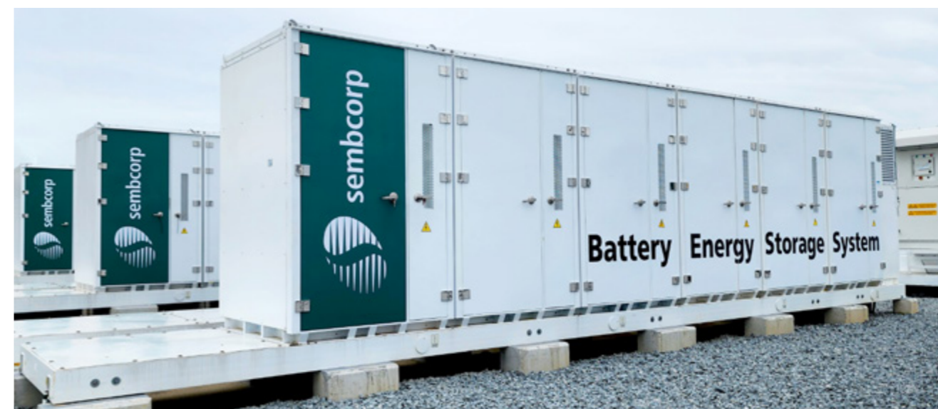
The Sembcorp ESS, Southeast Asia's largest ESS and fastest of its size to be deployed, was successfully commissioned in six months
