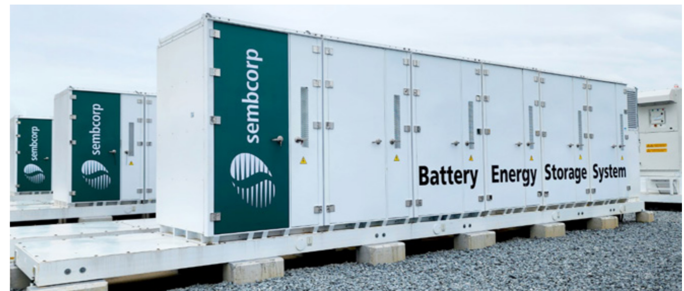
The Sembcorp ESS, Southeast Asia's largest ESS and fastest of its size to be deployed, was successfully commissioned in six months
