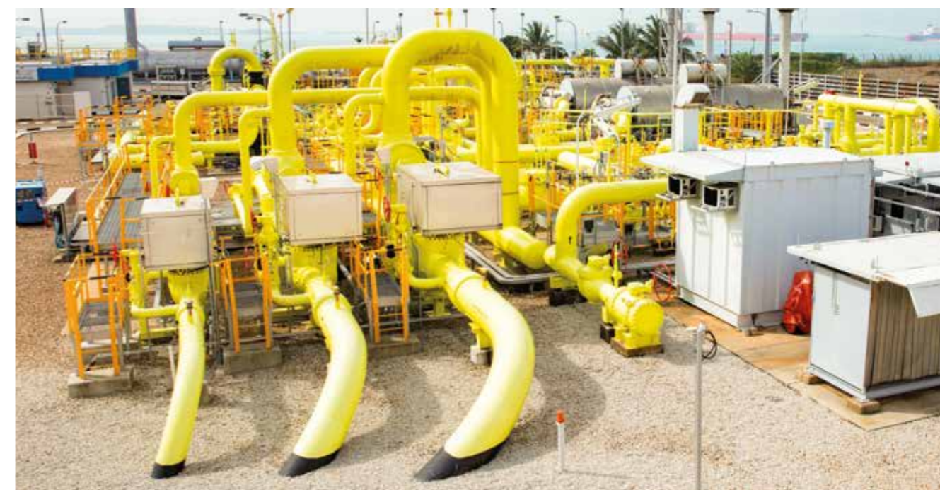
Sembcorp Gas Receiving Terminal on Jurong Island, Singapore
