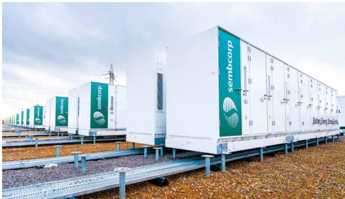
Battery energy storage system under construction at the Wilton International site on Teesside, UK
