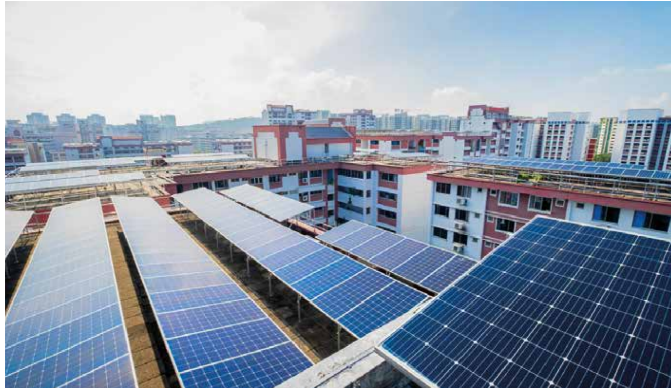
Solar photovoltaic (PV) systems installed on top of housing blocks as part of Singapore's SolarNova programme
