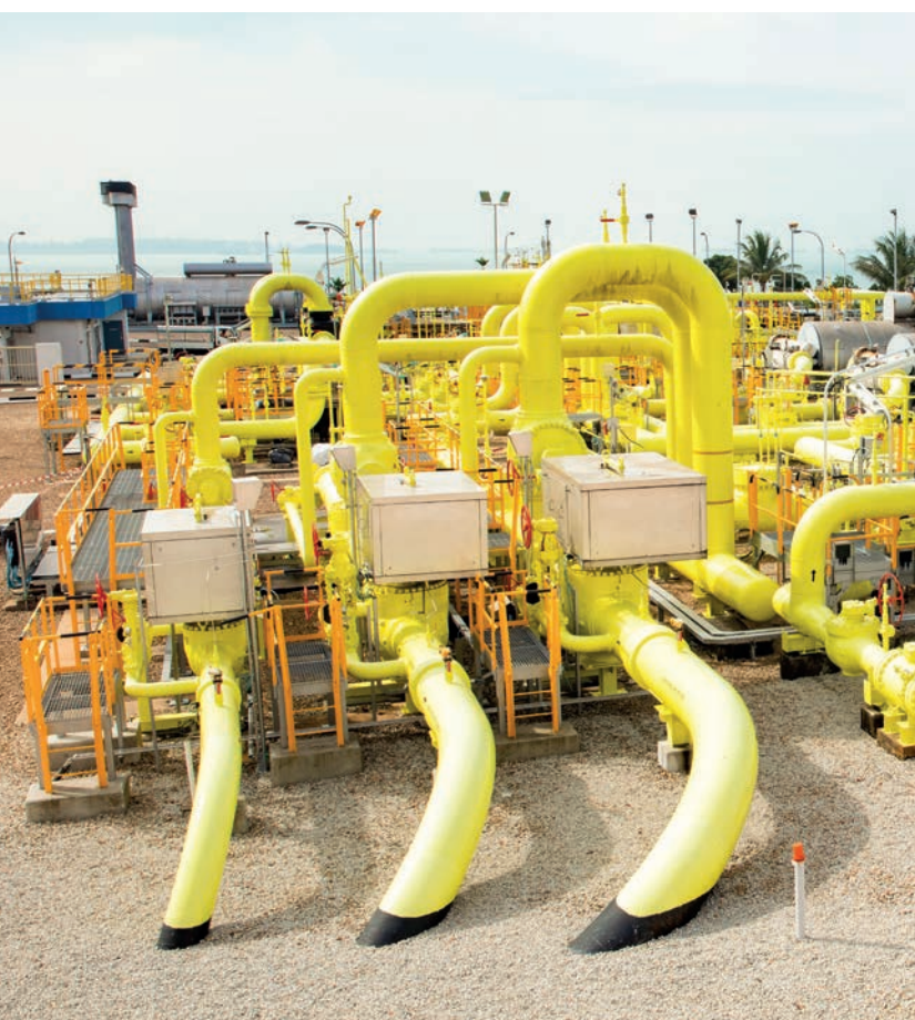
Sembcorp's Gas Receiving Terminal in Jurong Island, Singapore
