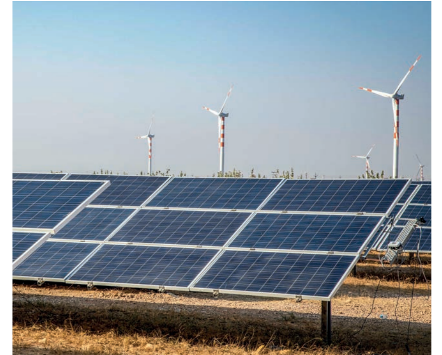
Sembcorp's hybrid renewables project in Rajasthan, India
