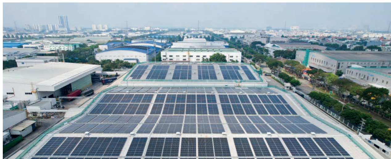
Rooftop solar panels installed on a tenant facility in Vietnam Singapore Industrial Park Binh Duong I, Vietnam
